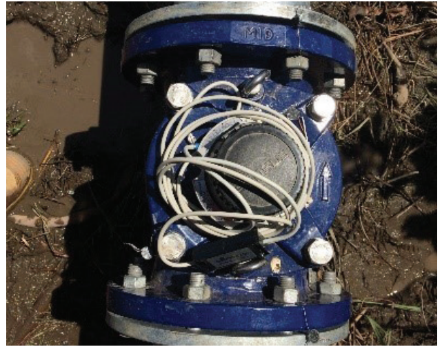
A Bermad Sensus water meter with a reed switch installed.
