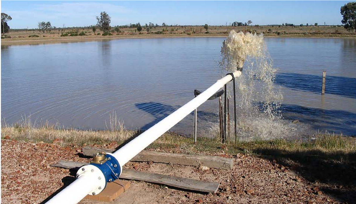
Open discharge meter with upturned end to keep pipe full of water.
