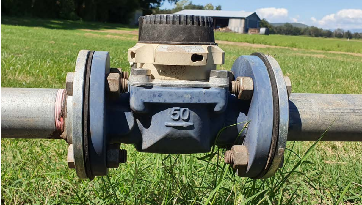
Example of an inline water meter.
